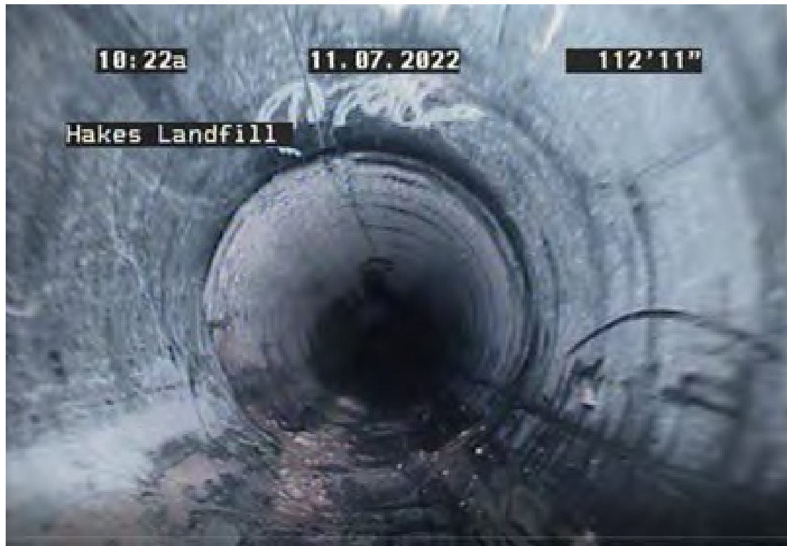
Photo showing minor accumulated sediment
