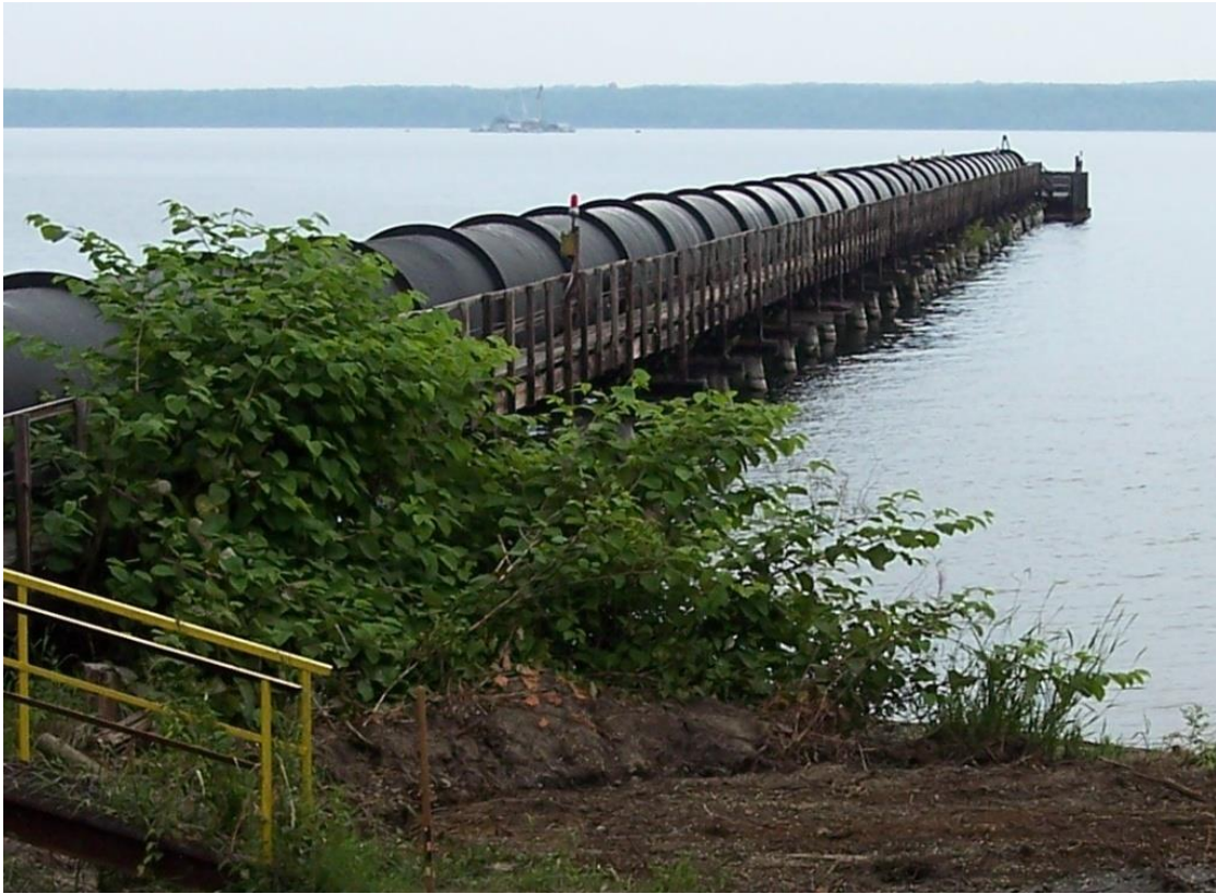
Figure 2-1 Unit 4 withdraws water from an elevated 7-ft diameter conduit that extends 650 from the west shore of Seneca Lake.
